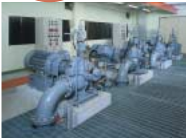
High-efficiency pump flow control
